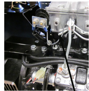
FUEL RETURN LINE CONNECTION
